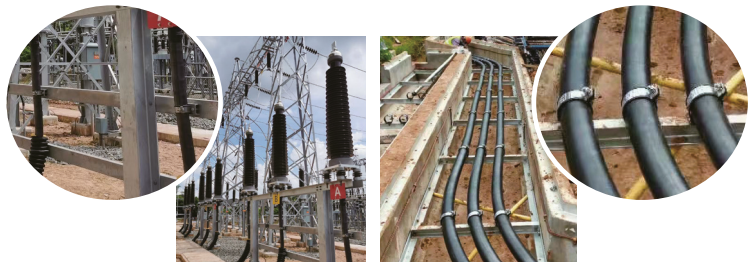
Power distribution substation
