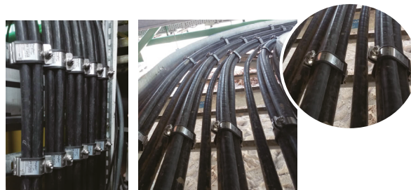
FPSO internal area
