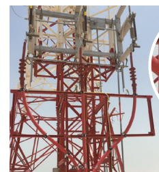
Power transmission tower
